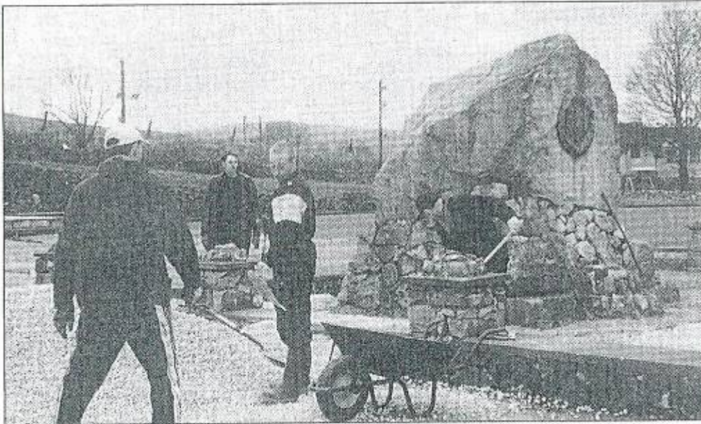
■ Hard at work on the Harpur Hill War Memorial site The monument was built 70 years ago.
